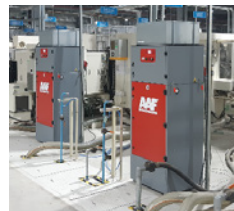
Compact dust collector on the manufacturing floor
